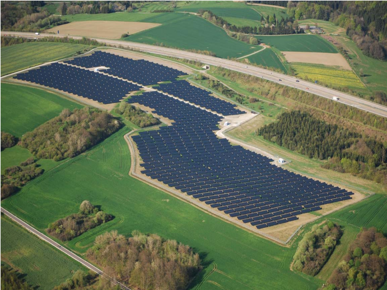
Agricultural site in Mehring, Germany: 3,450 kWp (modules supplied by First Solar)
