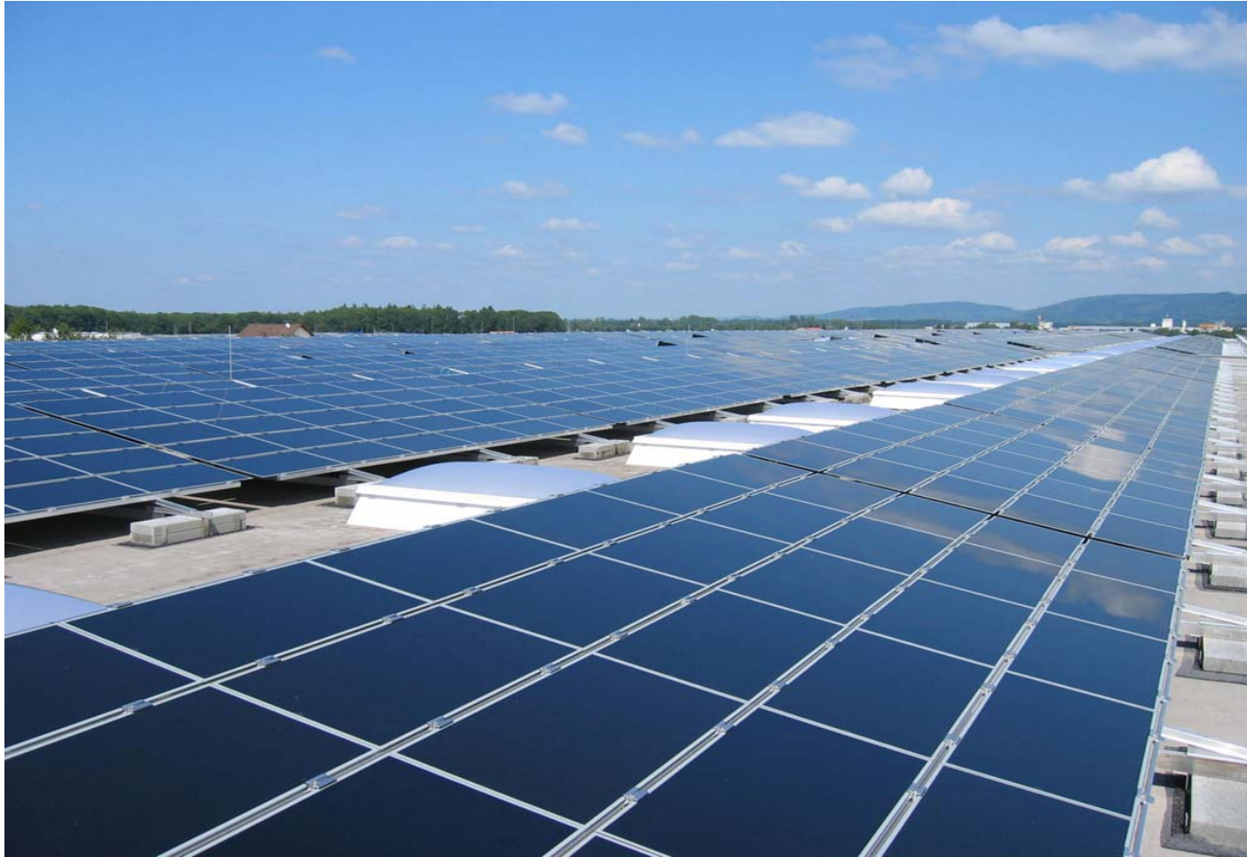
Logistic Center in Muggensturm, Germany: 1,800 kWp (modules supplied by First Solar)
