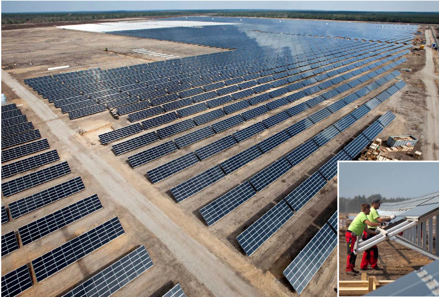
Former airfield in Lieberose, Brandenburg: 52,790 kWp (modules supplied by First Solar)
