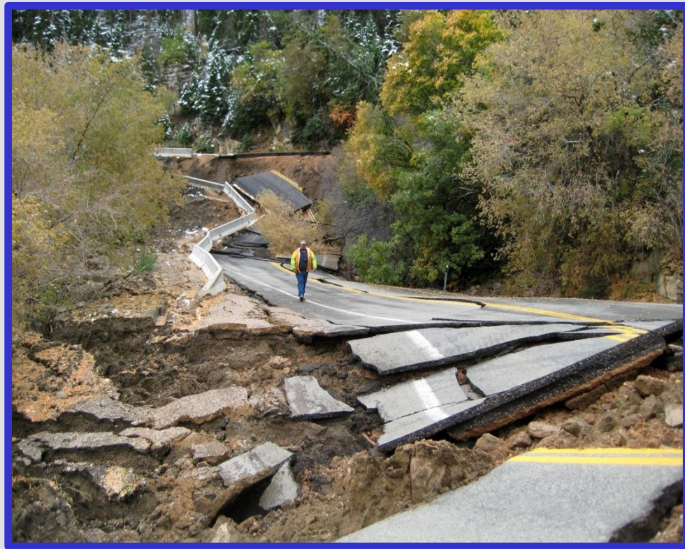
Route 14, Utah, USA after a landslide destroyed 400 m of road. (Image: MSNBC Photoblog, 2011)
