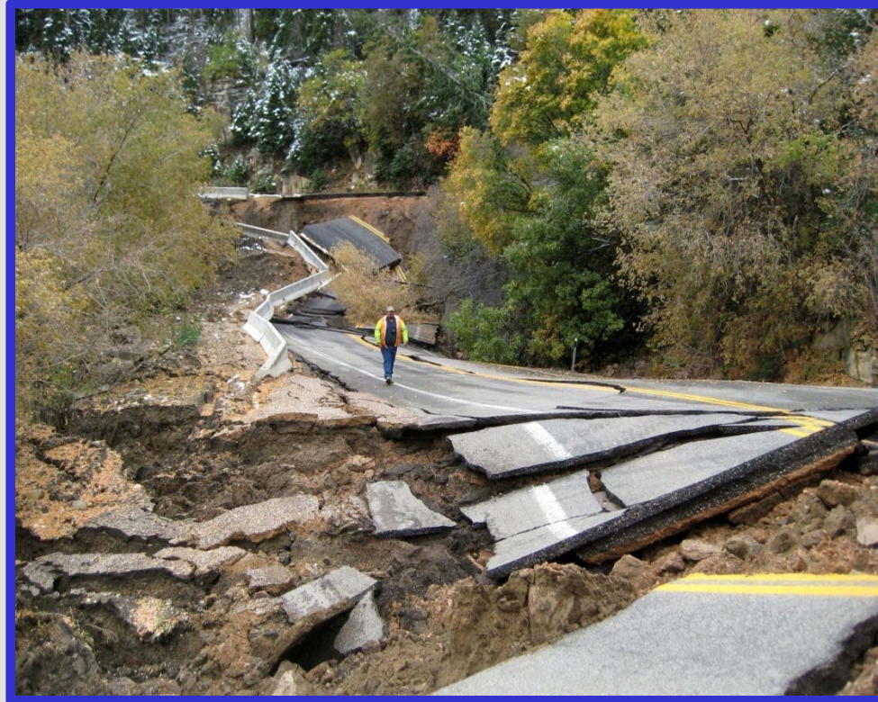
Route 14, Utah, USA after a landslide destroyed 400 m of road. (Image: MSNBC Photoblog, 2011)
