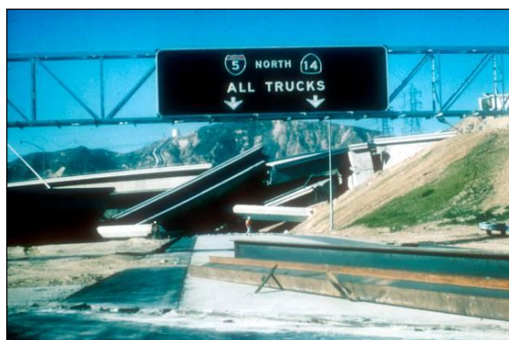
Earthquake damage to a bridge in USA, route 5 © USGS
