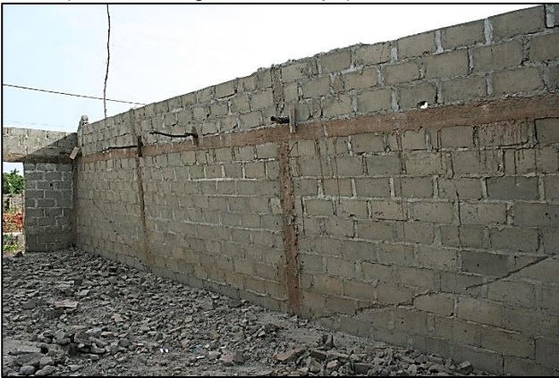
A wall damaged by monsoon weather in the Gambia.
