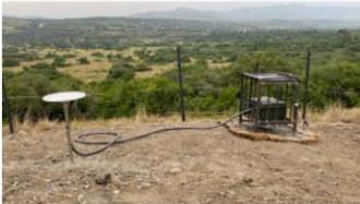
Installation of site UGN6 at the Queen's Pavilion (Uganda). Photo Credit: D. Sarah Stamps.
