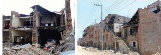
Figure 3. Fallen bricks near building from front wall collapse (left) and partial wall collapses (right), 2 earthquake (Credits: Anne Sanquini, (left), Bipin Shrestha (right), provided by Earthquake Engineering Institute)
